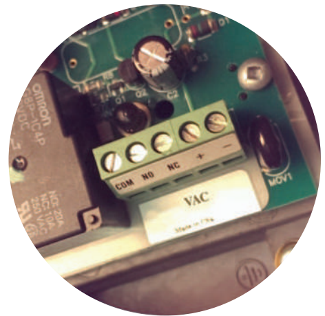
Figure R-7 DP-1C and DP-1D Terminal Block
